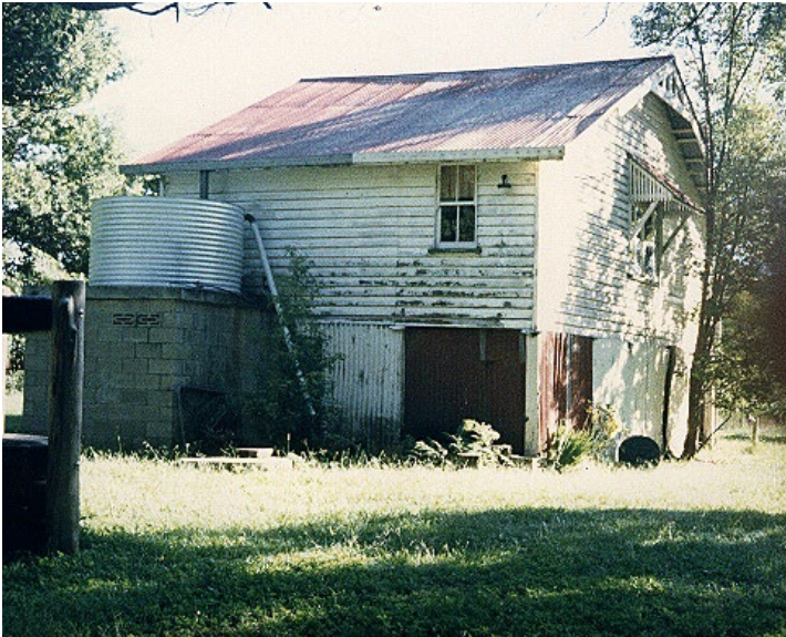
Left: 1996. The old school building was riddled with termites
